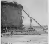
This tank under construction is one of four new ones being added to supplement motor Gasoline storage in the tank farm. Heavy workmen of Chicago Bridge make progress on tank No. 734, and the four are expected to be finished by the first of the year.
